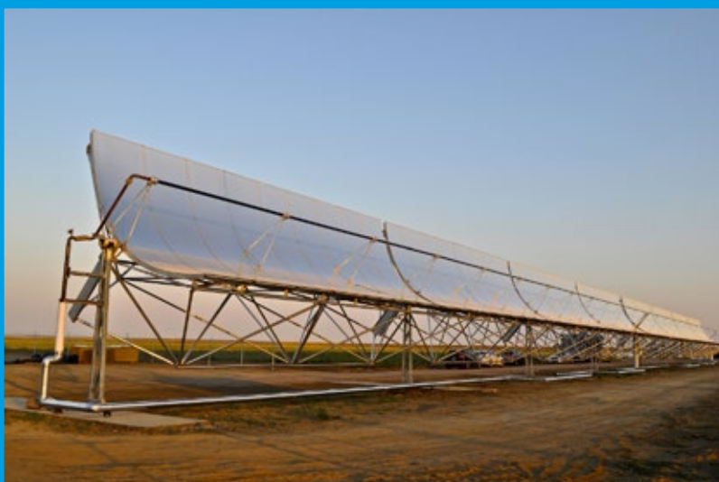
WaterFX Solar Water Desalination Plant's solar reflector
